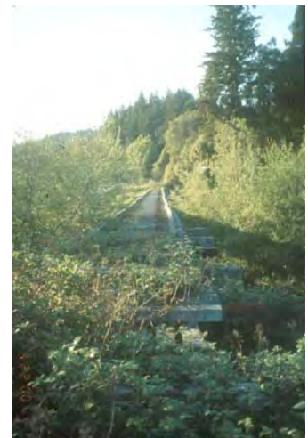
The Minor Creek Trestle is the most visible reminder of the A&M in Glendale.
