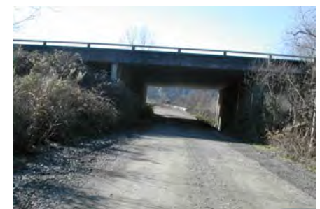
This private SR 299 undercrossing would be shared with industrial truck traffic in Glendale Alternatives D and E.
