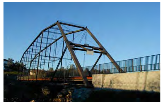
The historic Klamath River bridge was reinstalled for City of Folsom bikeway crossing at Lake Natoma. The retrofit included installation of the 54-inch high steel tubing fence for trail user safety.
