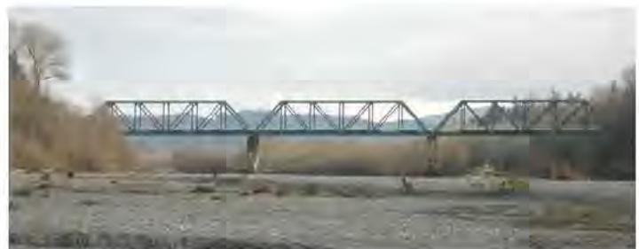
The 620-foot long Mad River bridge mostly consists of a steel truss superstructure much like that of the Hammond bridge.
