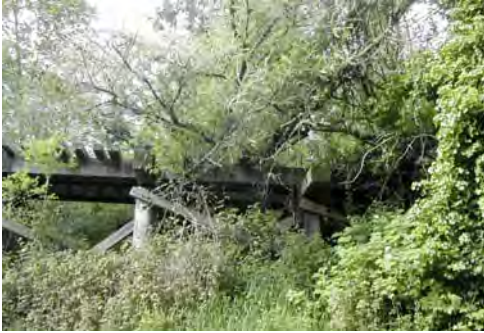
In less than five years since rail and tie were removed, much of the corridor is grown over, and several trees have fallen across trestles.
