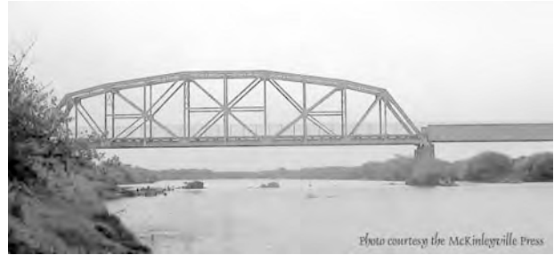
The Hammond Trail Mad River Bridge is just downstream, close to the beach, and of similar steel truss construction – and is substantially more corroded than the A&M bridge.
