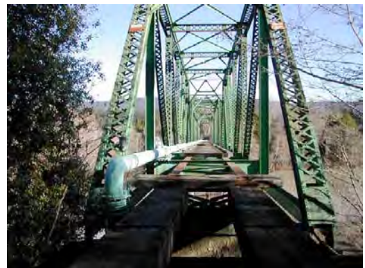
The Water District maintains a pipeline on the Mad River Bridge, and needs help maintaining the bridge.
