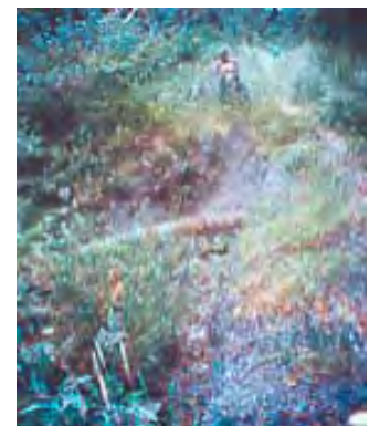
Lack of maintenance attention threatens the integrity of corridor infrastructure – and potentially that of downstream resources.
