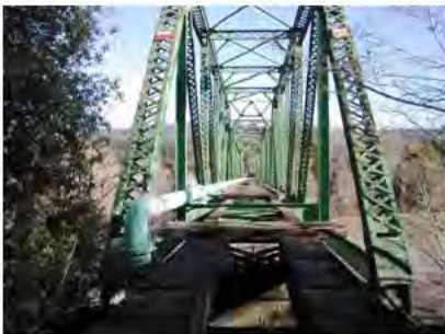
The A&M Mad River Bridge needs to be maintained because it also supports a HBMWD water line that serves Glendale and Blue Lake.
