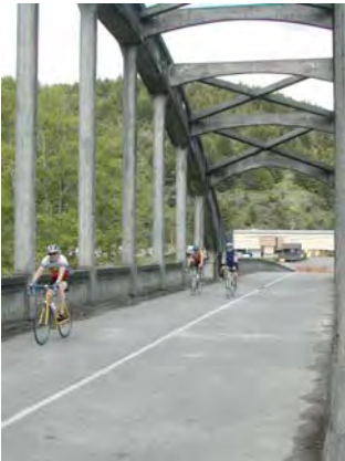
The North Fork Mad River Bridge in Korbelt is gateway to the popular ‘Butler Valley’ cycling route.
